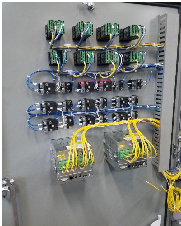
Fig. 4. The main control cabinet is placed out-of-cell to avoid radiation damage to the electronics. Cabling to the oven in cell is routed through the hot cell wall.
